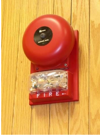
Figure: Audible and visual fire alarm
