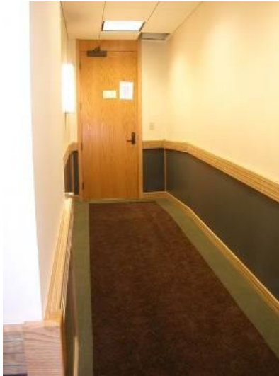
Figure: Common Error -This ramp provides access to the judge's bench from the rear; it lacks handrails. Additionally, the landing does not allow for someone to back up to get past the swing of the door or turn around if the door is locked or too difficult to operate.
