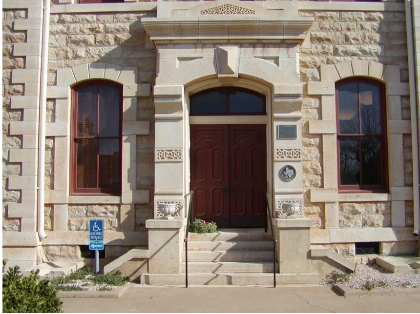
Figure: Inaccessible entrance with signage directing people to an accessible entrance.
