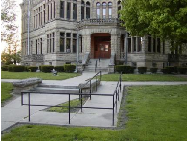
Figure: This exterior ramp is located along the same general path of travel as provided for the general public. However, while the ramp does provide handrails, it does not have edge protection.
