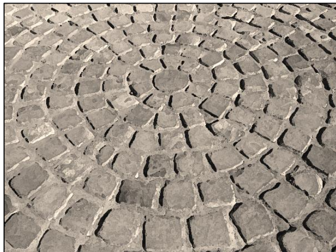
Cobblestones and other rough surfaces make wheelchair travel difficult and uncomfortable.
