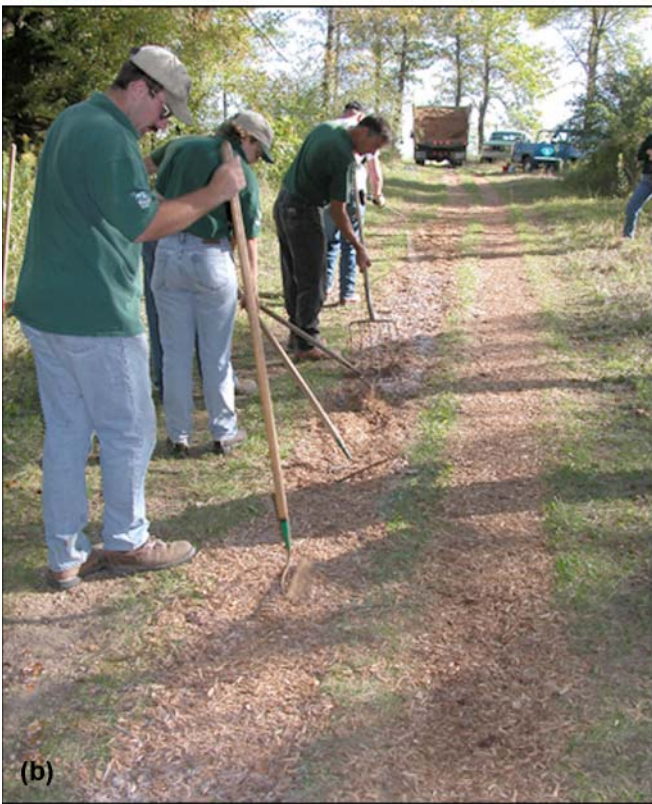
Figure 8—Installation of Soil-Sement surface on bridle path: (a) application of Soil-Sement by backpack-type sprayer; (b) trail crew mixed, leveled, and compacted the narrow trail filled with SEWF.
