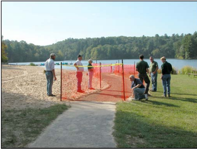
Figure 6—Completed beach path area looking west, shown with temporary barrier for 5-day SEWF curing period.
