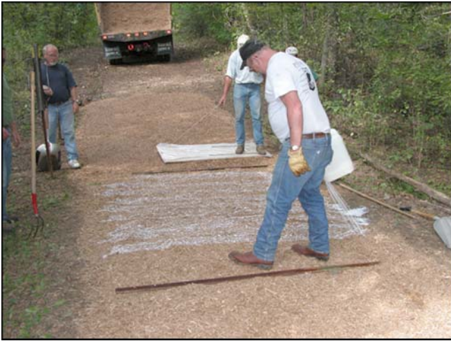
Figure 11—Treatment of wide bridle trail (site 2): spray application of Vitri-Turf in background and drip-bucket application of Soil-Sement in foreground. Note use of polyethylene-covered plywood for compaction and leveling of Vitri-Turf SEWF.
